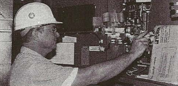
Local 120 Journeyman John Erbie, working for Johnson Controls
